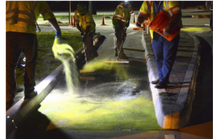
Researchers at Texas A&M University have designed a new bike lane that incorporates fluorescent paint. They also installed it on campus. (Texas A&M)
